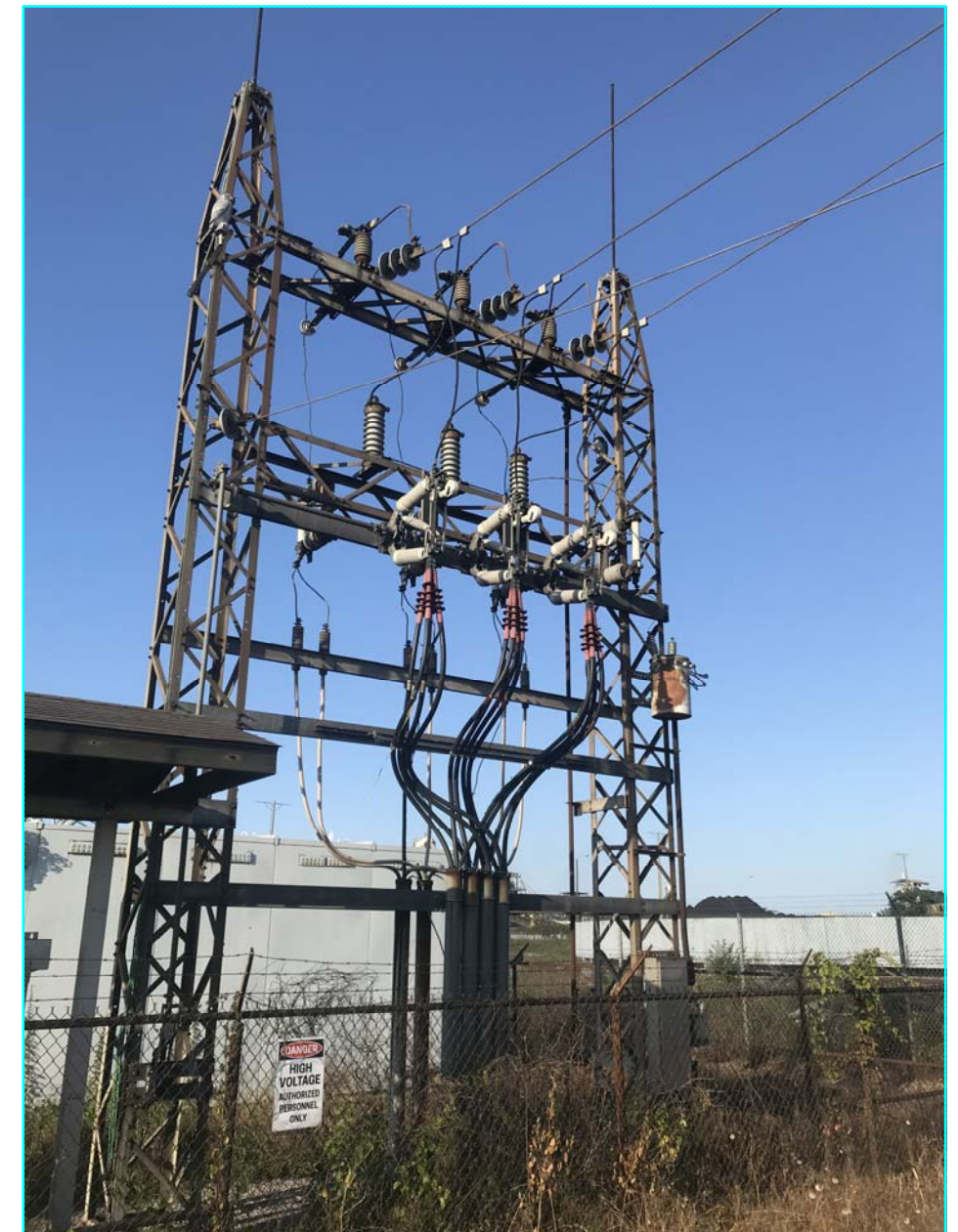
NORTH SIDE DEAD-END STRUCTURE
