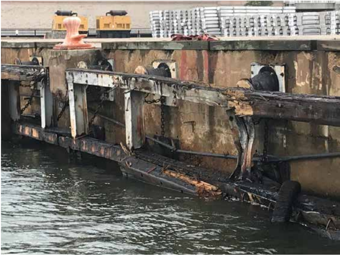
Berth 2 Fender System Allision Damage Between Bollards #6 & #7 – Looking Southwest
