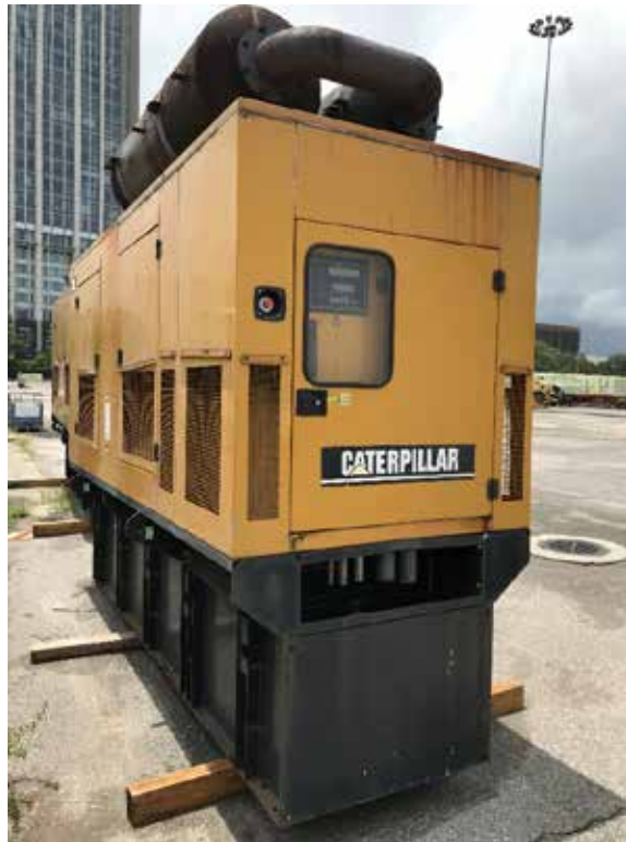
Paceco Crane #400 Generator – Engine Model: 3456 – Serial #: 7WG03870
