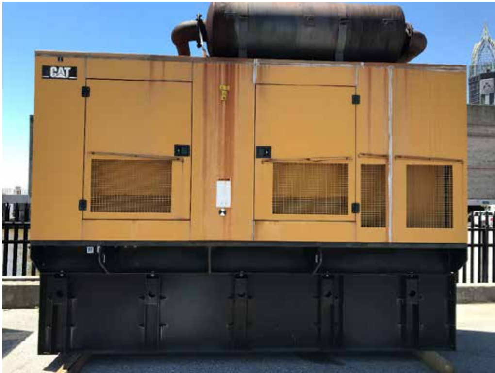
Paceco Crane #400 Generator – Engine Model: 3456 – Serial #: 7WG03856
