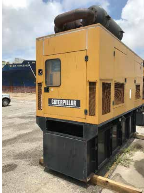
Paceco Crane #400 Generator – Engine Model: 3456 – Serial #: 7WG03856
