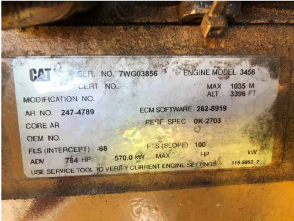
Paceco Crane #400 Generator – Engine Model: 3456 – Serial #: 7WG03856
