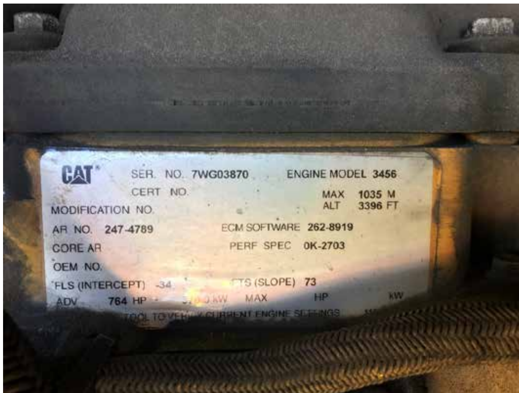
Paceco Crane #400 Generator – Engine Model: 3456 – Serial #: 7WG03870
