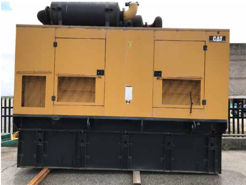
Paceco Crane #400 Generator – Engine Model: 3456 – Serial #: 7WG03870
