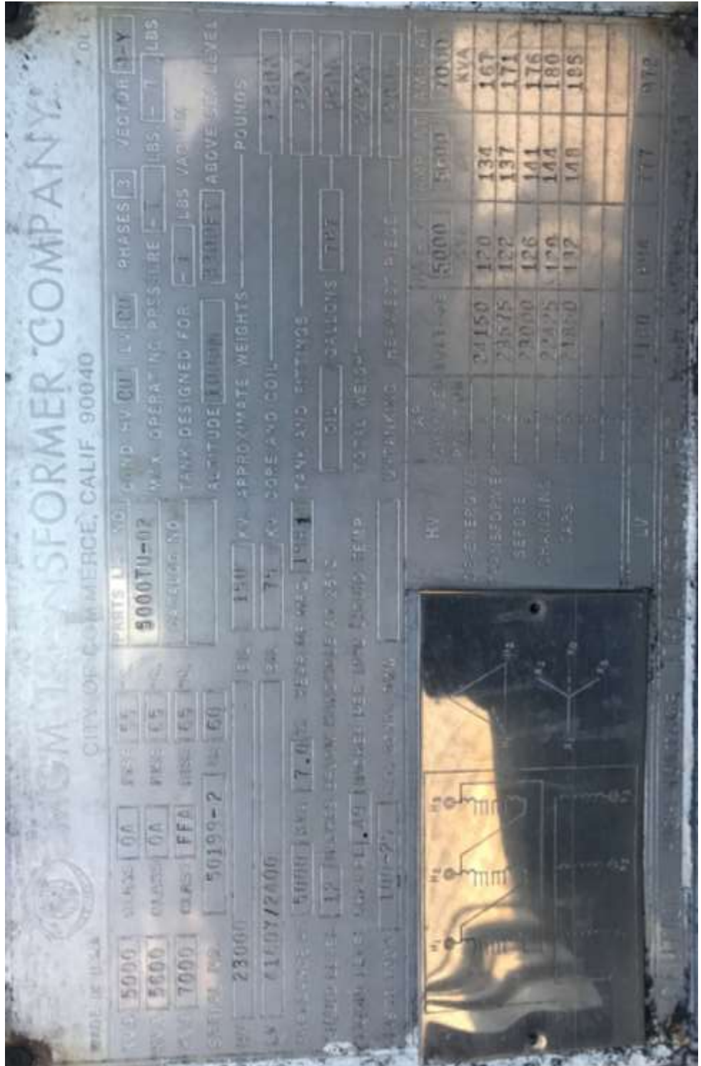
Substation Transformer for Northeast MCC Bldg.
