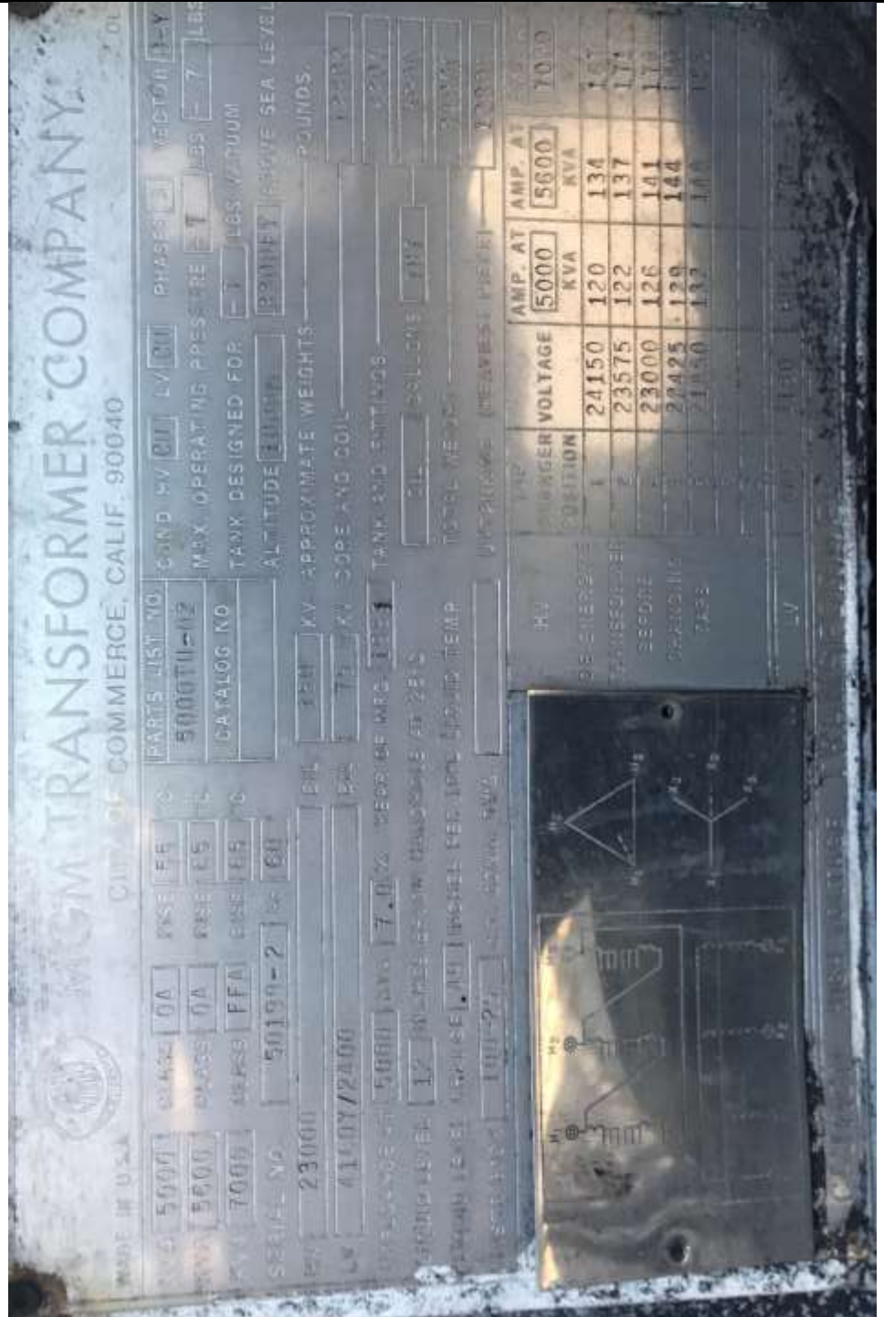
Substation Transformer for Northeast MCC Bldg.
