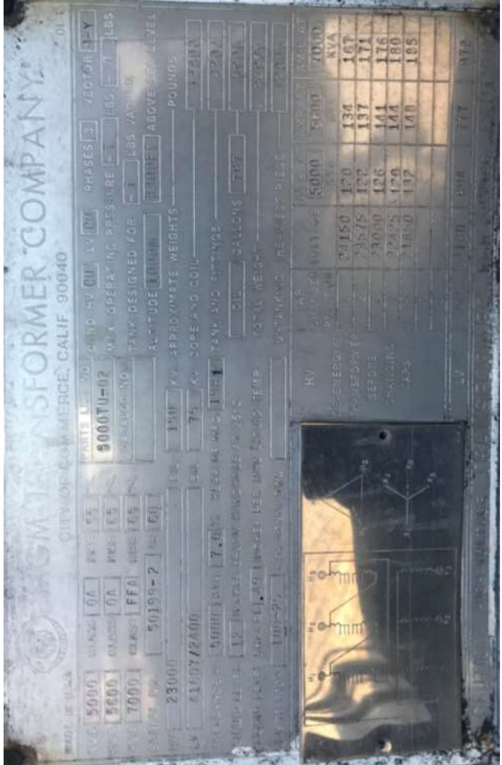
Substation Transformer for Northeast MCC Bldg.
