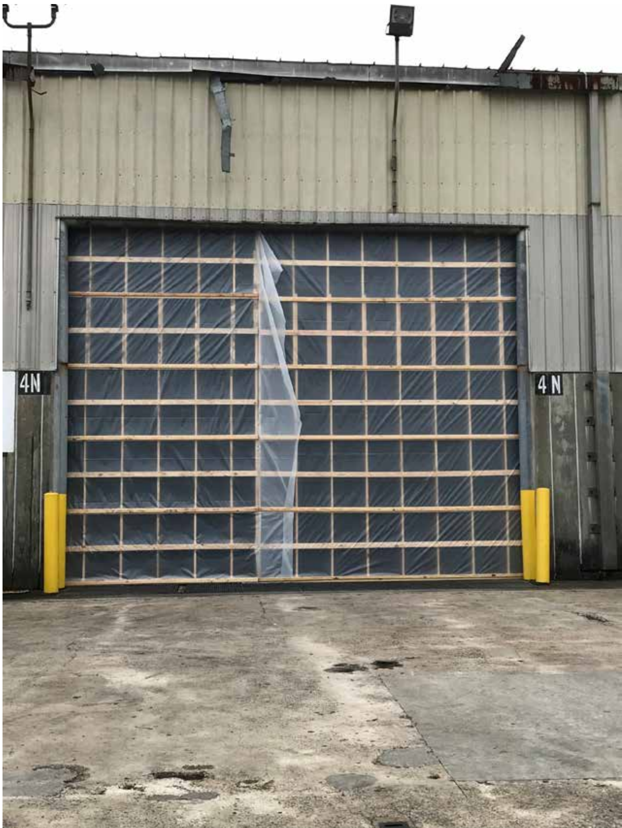
Typical Temporary Repairs North B-Door 2N, North B-Door 4N, North B-Door 7N and South B-Door 2N
