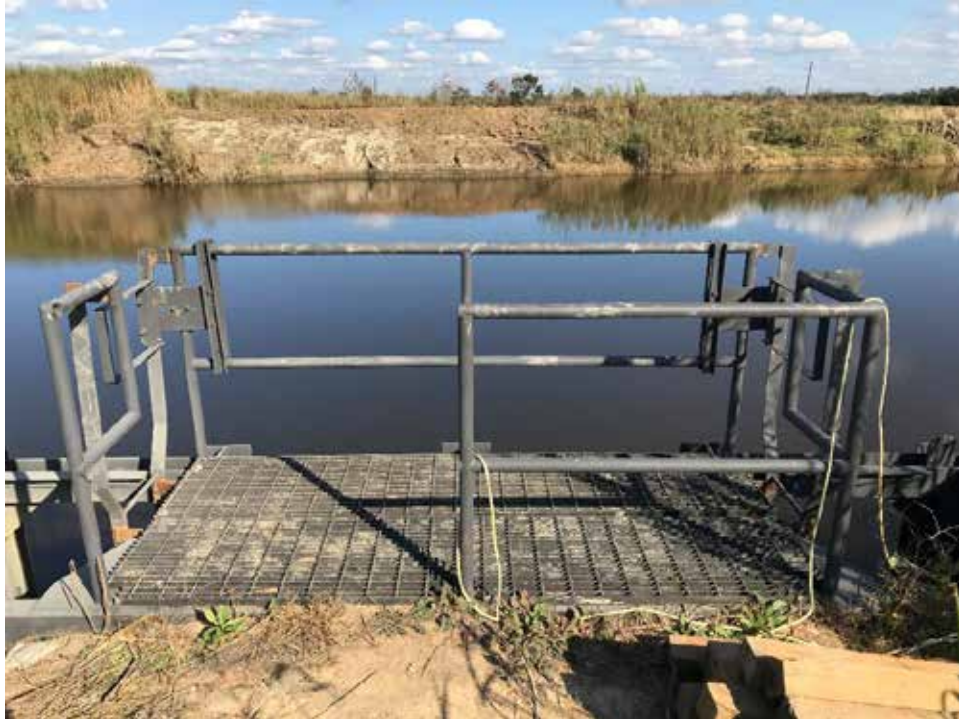
Existing grating, handrails, safety gates and walk thru ladders to be removed & reused
